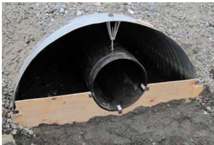
The first bulkhead is created after the pipe liner is inserted and before the grout is pumped in.
